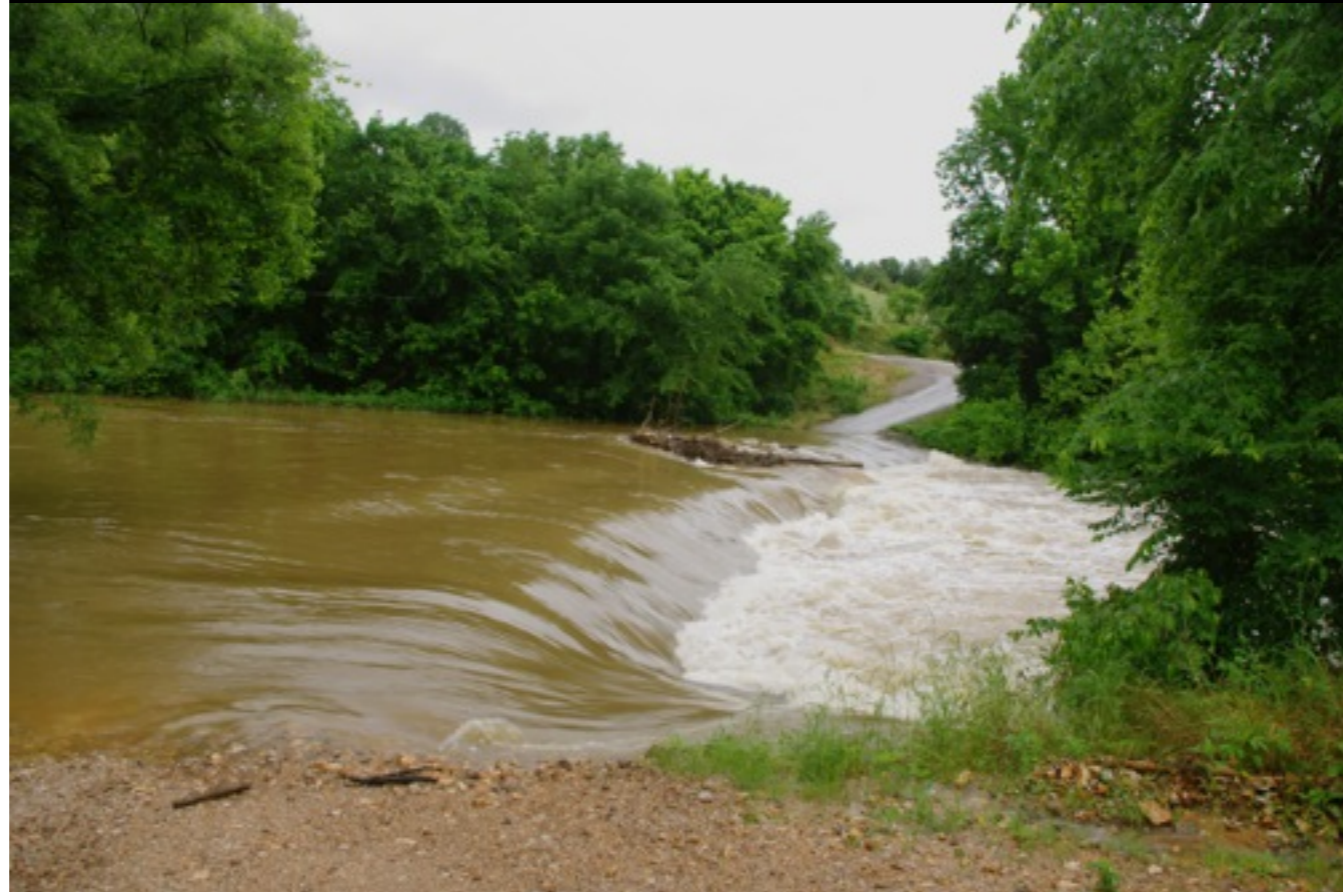
Low-water bridge overtopped by intense summer runoff
