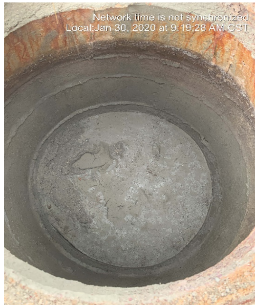
Photograph 2: Manhole leading to Pond 1 was filled with concrete to stop any future waste from being added to the ponds from the hog houses.
