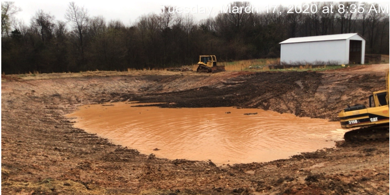
Photograph 30: Removal of solid waste from Pond 1 continued. Additional rainfall resulted in additional liquid waste in Pond 1.
