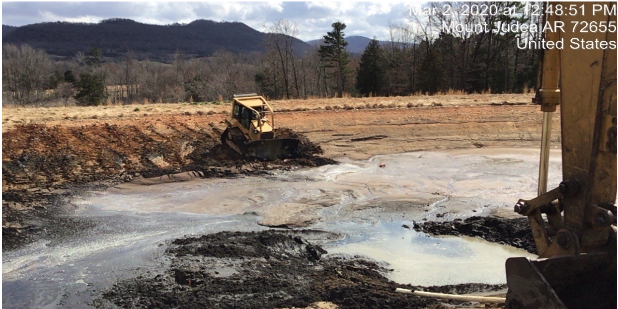
Photograph 21: Solid waste in Pond 1 being pushed toward excavator so it may be loaded into dump trailers and transported to a landfill.
