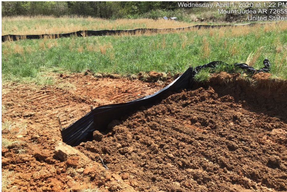
Photograph 40: Silt fence was placed across breach in the levee of Pond 1 to ensure no sediment was allowed to erode during rain events.
