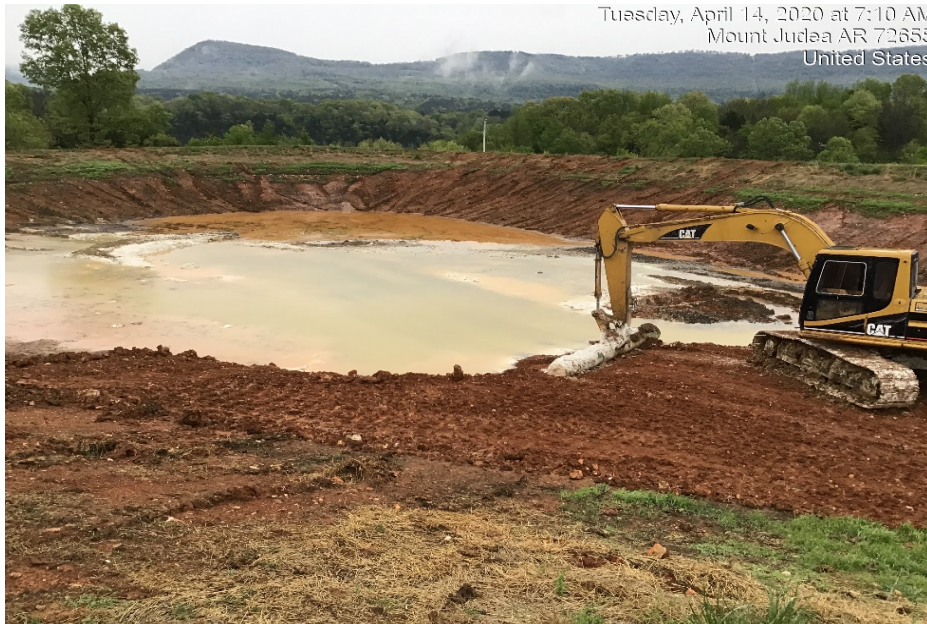
Photograph 49: Additional rainfall resulted in more liquid waste in Pond 2.
