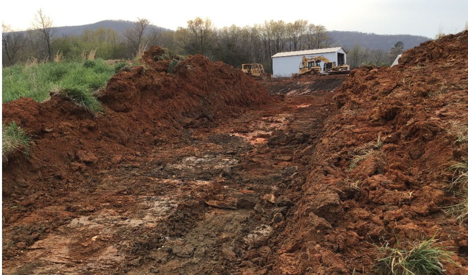
Photograph 37: Levee of Pond 1 was cut to ensure rainfall does not result in additional liquid waste to be removed.
