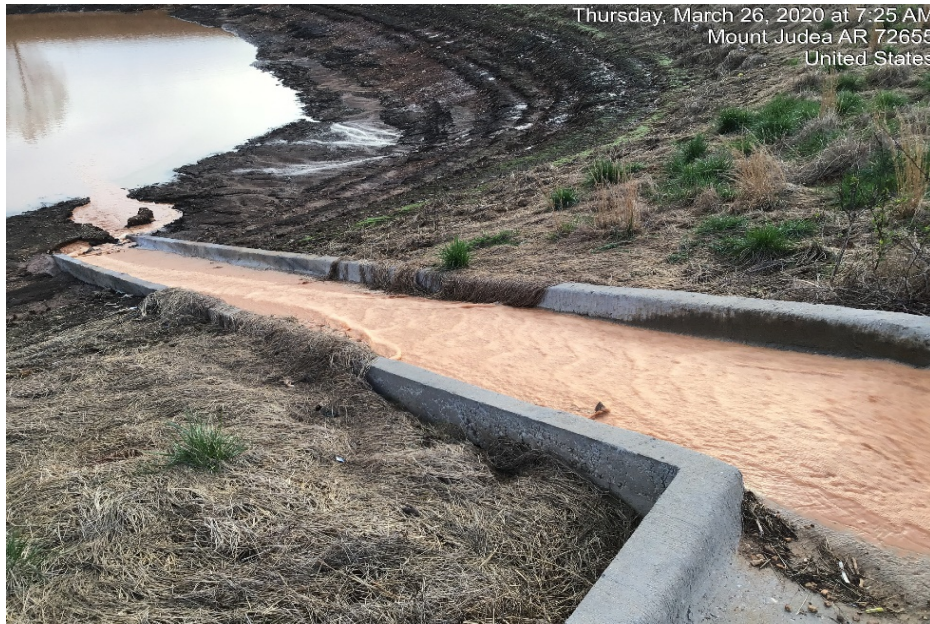
Photograph 33: Liquid waste due to rainfall was pumped from Pond 1 to Pond 2.
