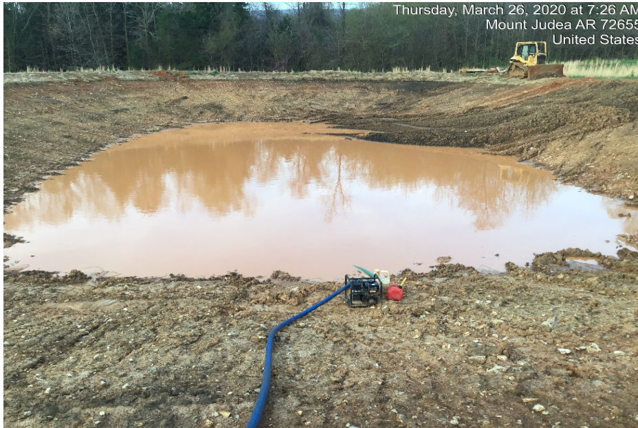
Photograph 34: Liquid waste due to rainfall was pumped from Pond 1 to Pond 2.
