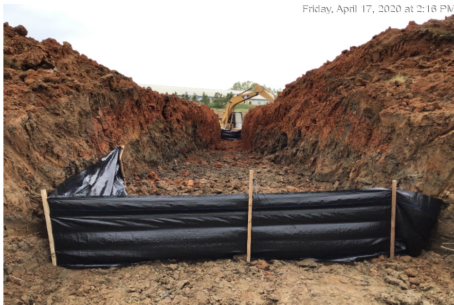
Photograph 52: Levee of Pond 2 breached, and silt fence was placed to ensure no sediment was allowed to erode during rain events.
