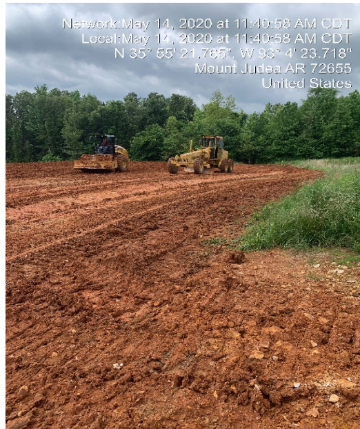
Photograph 59: Diversion ditch was created to ensure all runoff of adjacent areas does not travel across the site.
