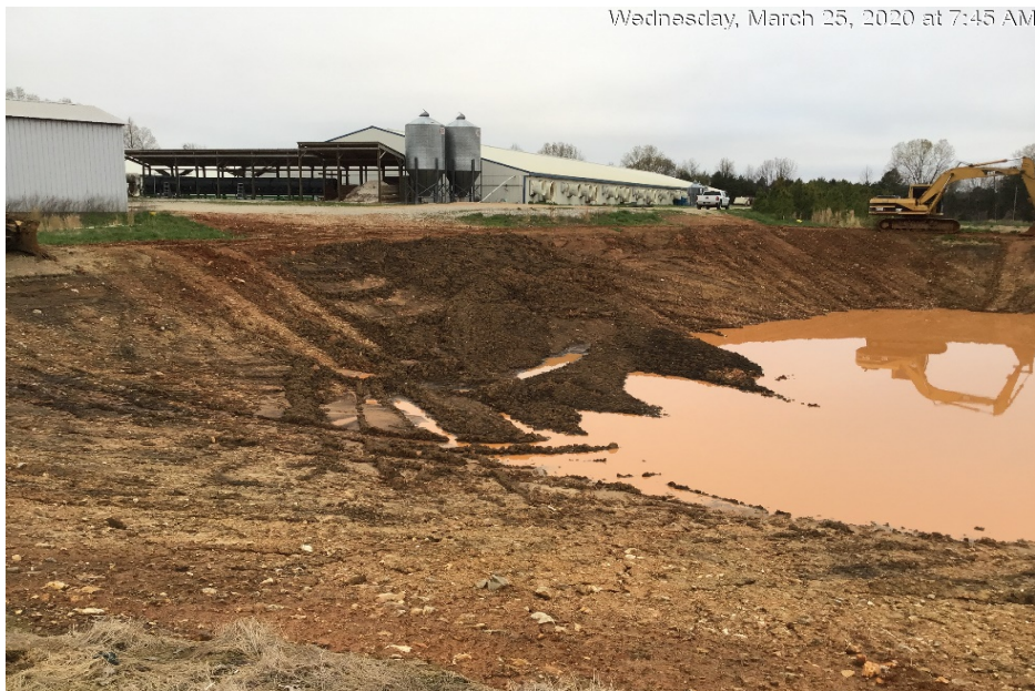
Photograph 32: Removal of solid waste from Pond 1 continued. Additional rainfall resulted in additional liquid waste in Pond 1.
