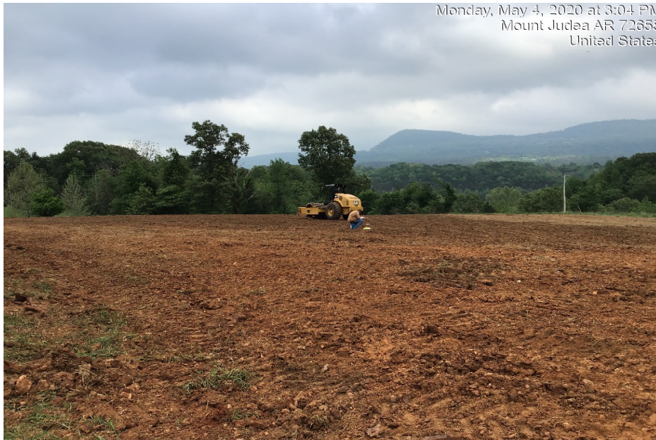
Photograph 57: Material being placed in compacted lifts over Pond 2 continued, and soil density tests continued.
