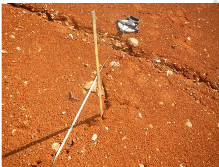
Figure 1 Liner cracks (from inspection report visit by ADEQ, Tony Morris 7/23/13)
