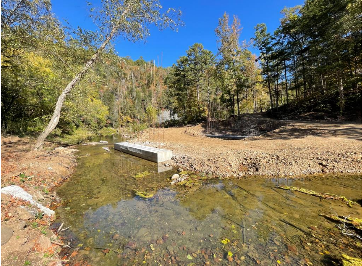
Figure 6. Newton county road 252 crossing on Cave Creek in Gene Rush Wildlife Management Area under construction.
